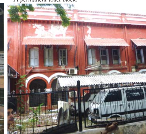
Temporary van shelters and corrugated iron shades for windows. Note the state of the walls.
