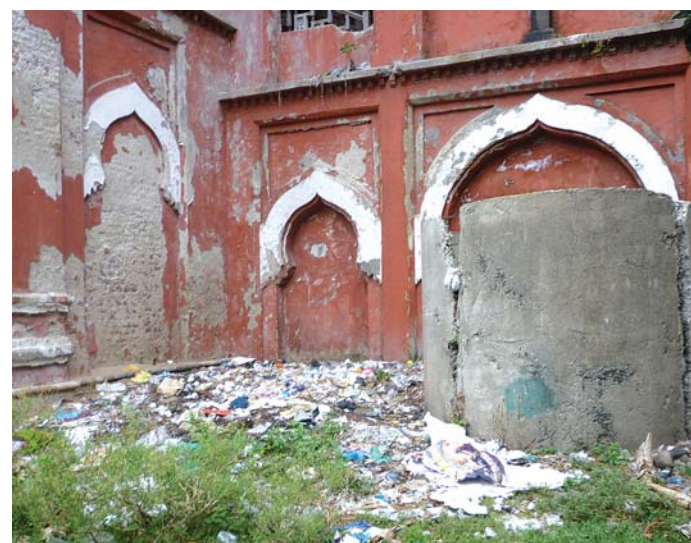
A garbage dump lying unintended beside deteriorating walls.
